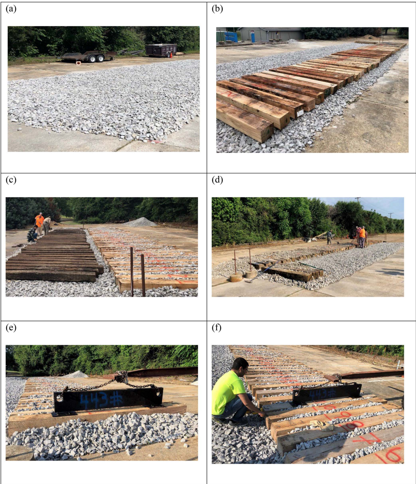
Figure 1.—(a) Ballast rock bed, (b) freshly cut green ties installed on the ballast, (c) installation of legacy ties on the ballast, (d) installation of ballast between each of the ties, (e) 200-kg (434-lb) weight constructed and used to simulate the load of the rails on each tie, and (f) measurement of acoustic velocity of a given tie (identification number 11) while in the fixed boundary condition.
