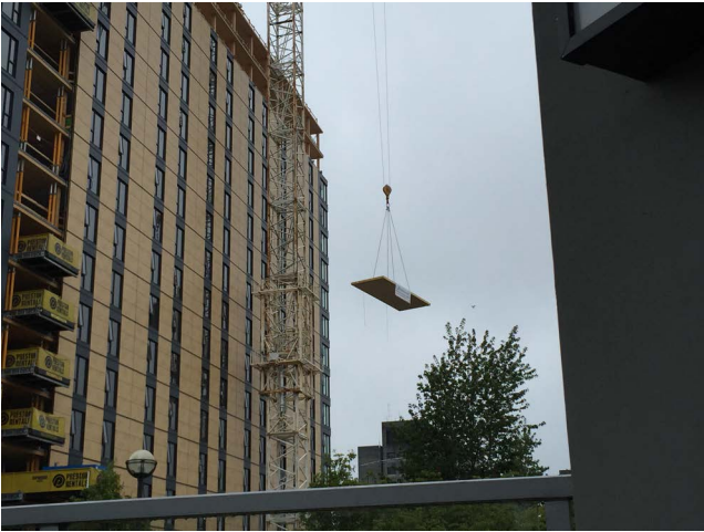
A panel is being lifted into place during construction of the 18-story Brock Commons Tallwood House student residence at The University of British Columbia.
