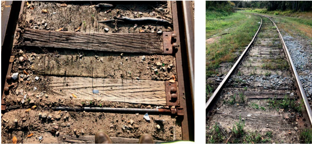
Figure 6.—Test ties in track (left) showing poor ballast and radius track (right).
