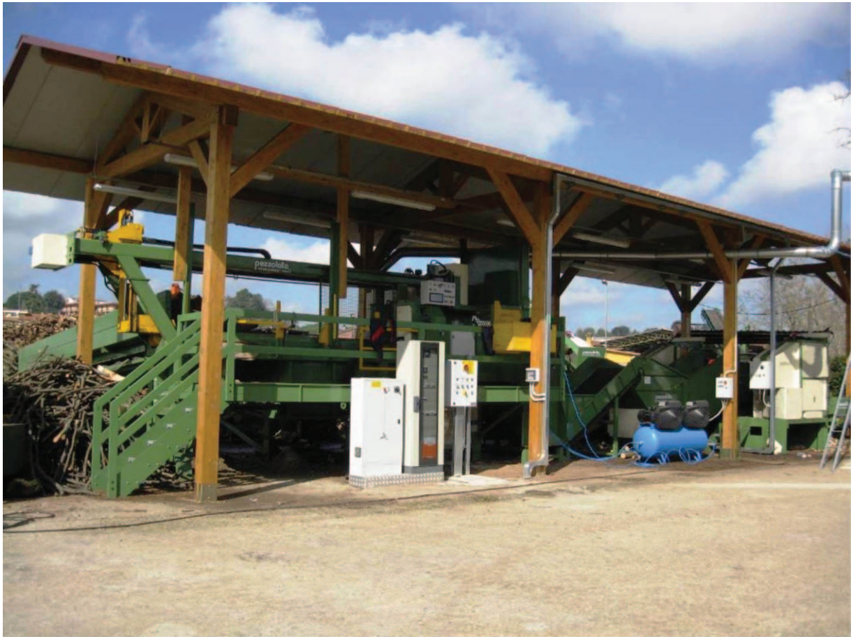
Figure 1.—Industrial firewood processor, showing the in-line layout, stationary installation, and electric power panels (Operation 4).
