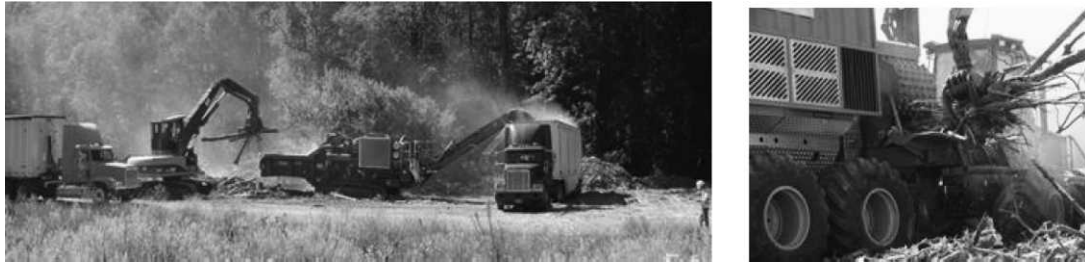
Figure 1.—Field processing of logging slash in southwest Oregon. (Left) Peterson-Pacific horizontal grinder. (Right) Bruks horizontal chipper.
