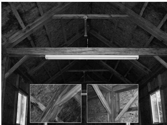
Figure 1.—The post-and-beam building constructed in 2008 for the Mid-South Forestry and Equipment Show.
