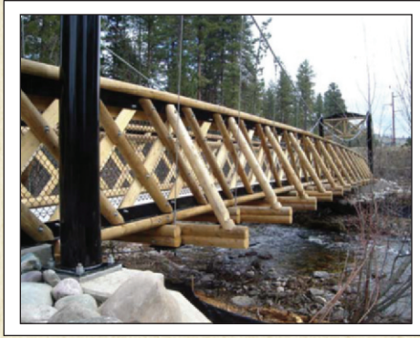
The Rattlesnake Creek bridge near Missoula, Montana, was built using 6-inch-diameter lodgepole pine from a forest in Idaho to demonstrate the effective use of trees killed by the pine bark beetle.
